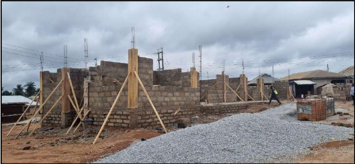
Annex 2: 1 No. 2-Unit KG Block at Ejisu Experimental Basic School - Ejisu (On-going)
